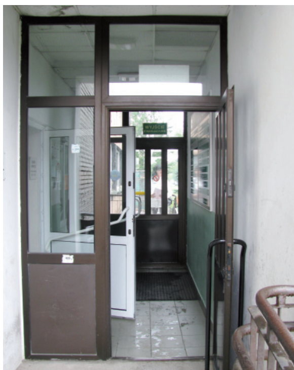
Picture 4 Entry door impeding wheelchair access
