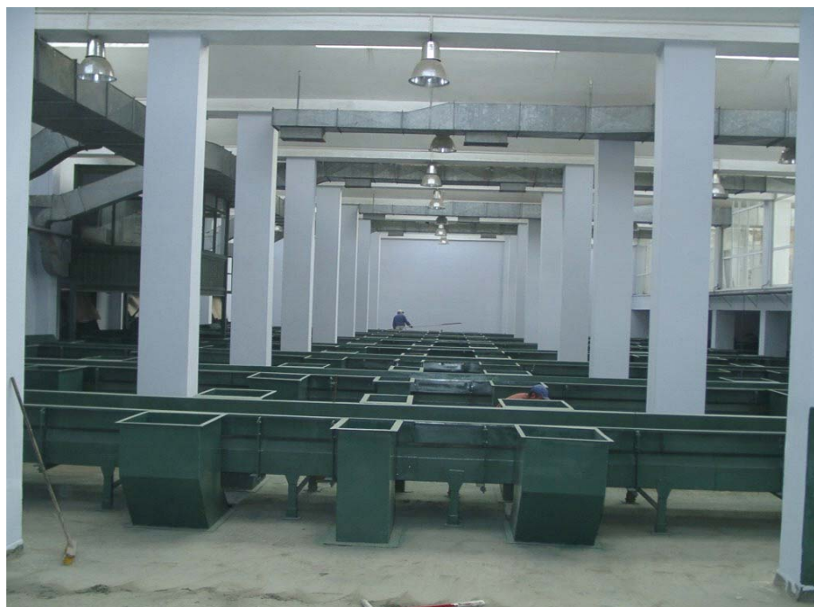
Figure 9: Packaging Waste Separation Facility in Ankara
